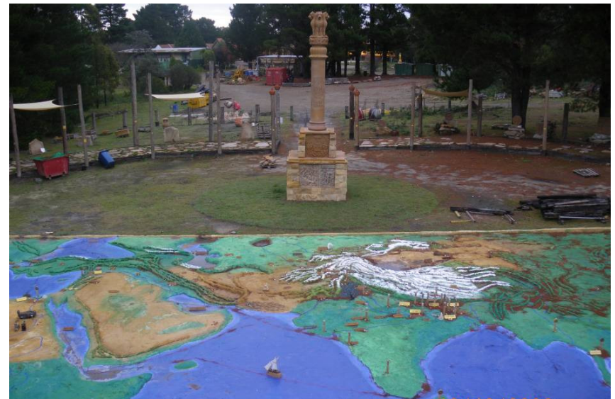
Ashoka Pillar, topographical map and sculpture garden with the walking meditation pathway under construction – May 2009
